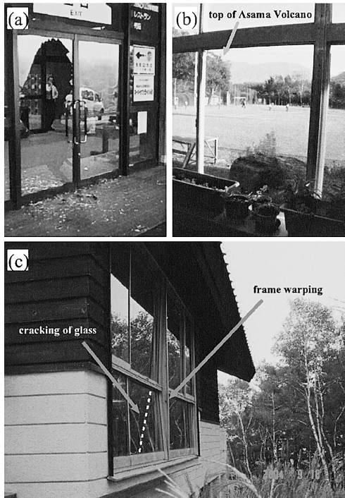
Fig. 2. Photos of (a) glass breakage at the Asama Volcano Museum taken by Kyodo News, (b) a view from a broken window at Tashiro Primary School and (c) a glass crack at the Asama Memory House taken by M. Enomoto.
